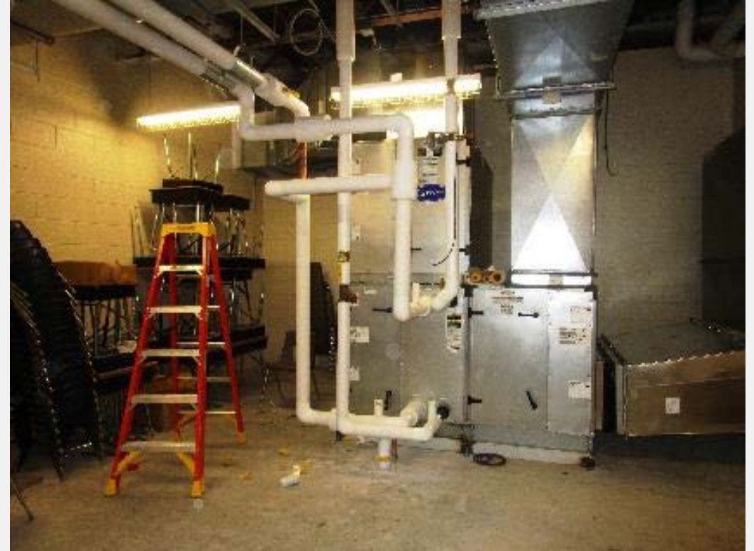
Elementary – Gymnasium – AHU 1
